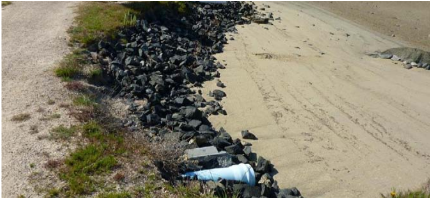
Lack of foreshore vegetation, foreshore erosion and exposed storwater pipes
