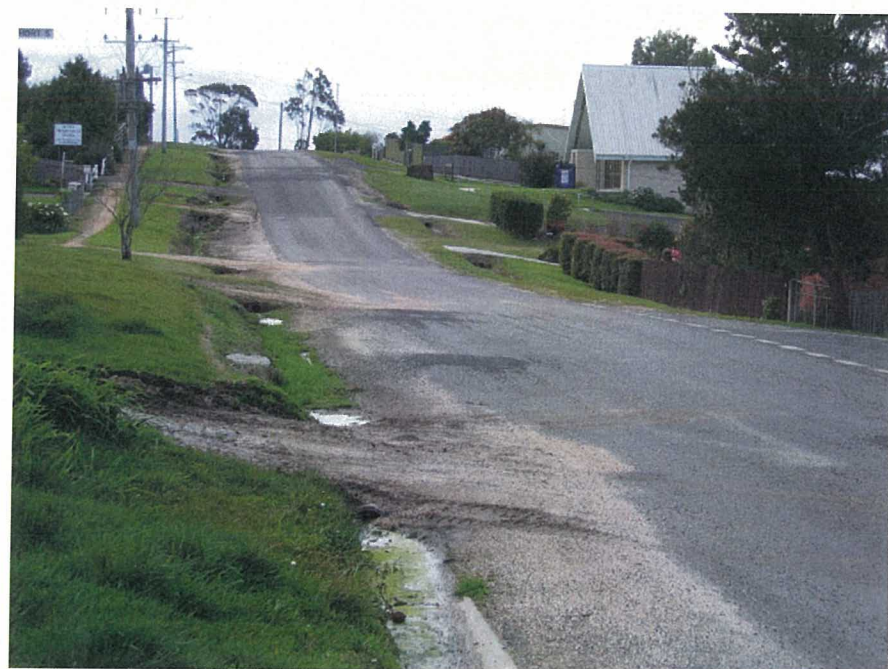
Figure 22: Some local roads have poor drainage & surfaces
