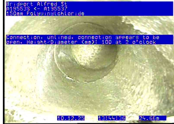
A195273_09433cea-8256-4cb9-a744-edf1d618daae_20251210_134451_309.jpg, 00:03:33, 24.66 Connection, unlined, connection appears to be open, Height/Diameter (mm): 100 at 2 o'clock
