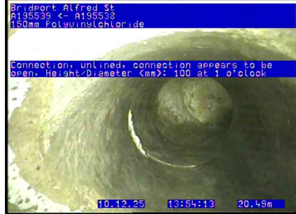
A195272_db9302ab-87b0-4f4a-94d5-0a722373f54a_20251210_135428_920.jpg, 00:03:03, 20.49 Connection, unlined, connection appears to be open, Height/Diameter (mm): 100 at 1 o'clock
