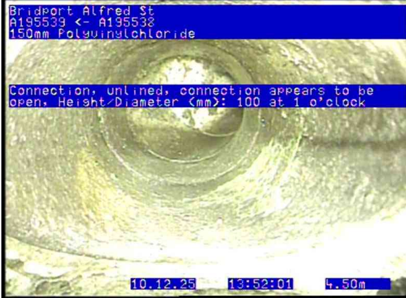
A195272_f3b1a85b-d2ee-4719-b704-748be81b6909_20251210_135217_133.jpg, 00:01:00, 4.50 Connection, unlined, connection appears to be open, Height/Diameter (mm): 100 at 1 o'clock
