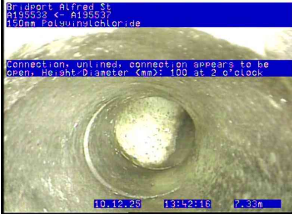
A195273_4ae9c2da-4e33-4969-bc3d-1252b0434f7b_20251210_134231_561.jpg, 00:01:22, 7.33 Connection, unlined, connection appears to be open, Height/Diameter (mm): 100 at 2 o'clock
