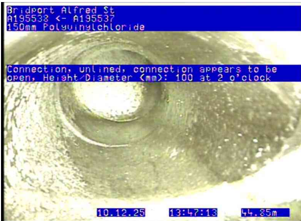
A195273_fbf5721f-5823-4cd0-89ae-2e16367f13d3_20251210_134728_841.jpg, 00:06:02, 44.85 Connection, unlined, connection appears to be open, Height/Diameter (mm): 100 at 2 o'clock
